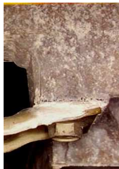
Fig. 4. Magnesium alloy casting fastened to a steel bracket using a coated steel bolt. The interface between the steel bracket and the magnesium casting surface is prone to galvanic corrosion.
